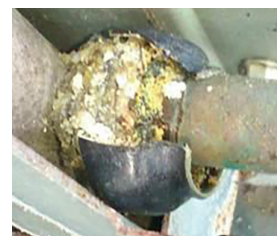
Galvanic corrosion under the plastic sleeve.
